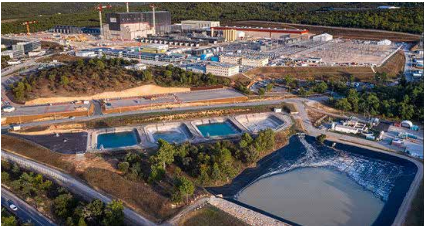
An aerial view of the construction site of ITER and the surrounding complex at Saint-Paul-lès-Durance, France. Construction at the site began in August 2010, and is not expected to be completed until at least 2025. Photo by Matjaz Krivic
